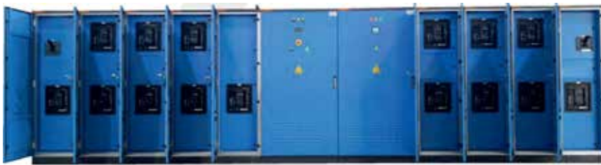
Indoor Type Distribution Board
