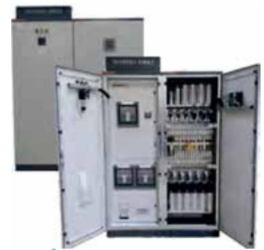
Indoor Type LV Distribution and Compensation Panel
