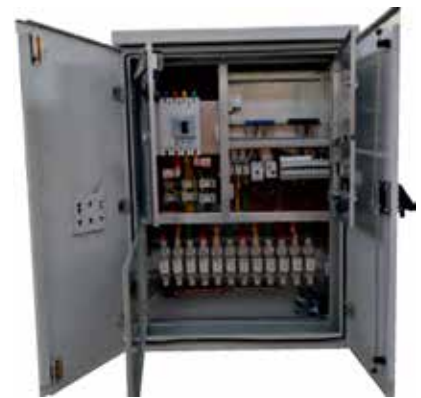
Outdoor Type Distribution Board
